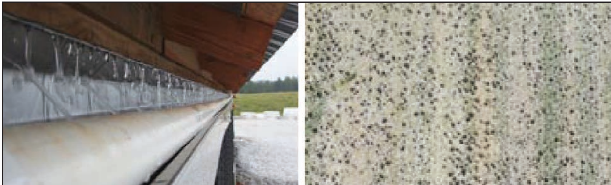
For most efficient and effective pad cooling, pads must be thoroughly wet. For recirculating pad systems, it is important to check headers regularly to be certain there are no plugged holes in the discharge pipe. Photo at left above shows properly functioning header. Right photo shows a thoroughly clogged pad. Flushing pads with water and using one of the widely available cleaning products helps prevent pad clogging. Clogged pads raise static pressure, reduce fan cfm's and wind speed, and reduce both real and wind-chill effective cooling.
