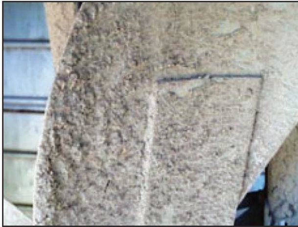
Above photo is a close-up view of a fan blade that has not been cleaned for several weeks. The dust and dirt build-up changes the aerodynamics of the blade and puts additional drag on the blade, severely reducing fan performance.
