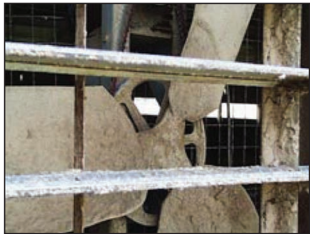
Above photo shows how dirty fan blades and shutters can get in just a short time. Build-up of dust and dirt on shutters and blades can reduce fan performance by as much as 30% in real world applications.
